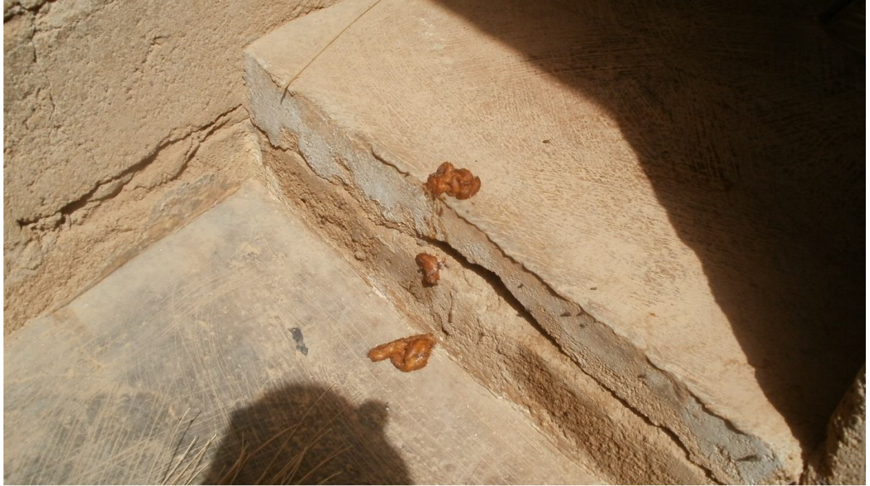
PICTURE I: CONDITION OF THE TOILETS BEFORE THE WORKSHOP
