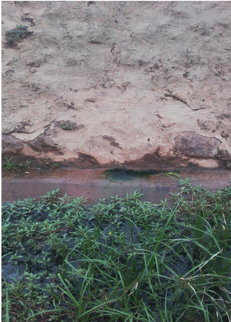
Figure 4.2. Second Seepage Area of Goronyo Dam
