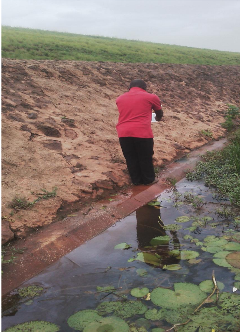
Figure 4.1. First seepage area of Goronyo Dam
