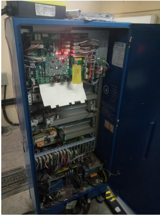
Lift control sytem board box
