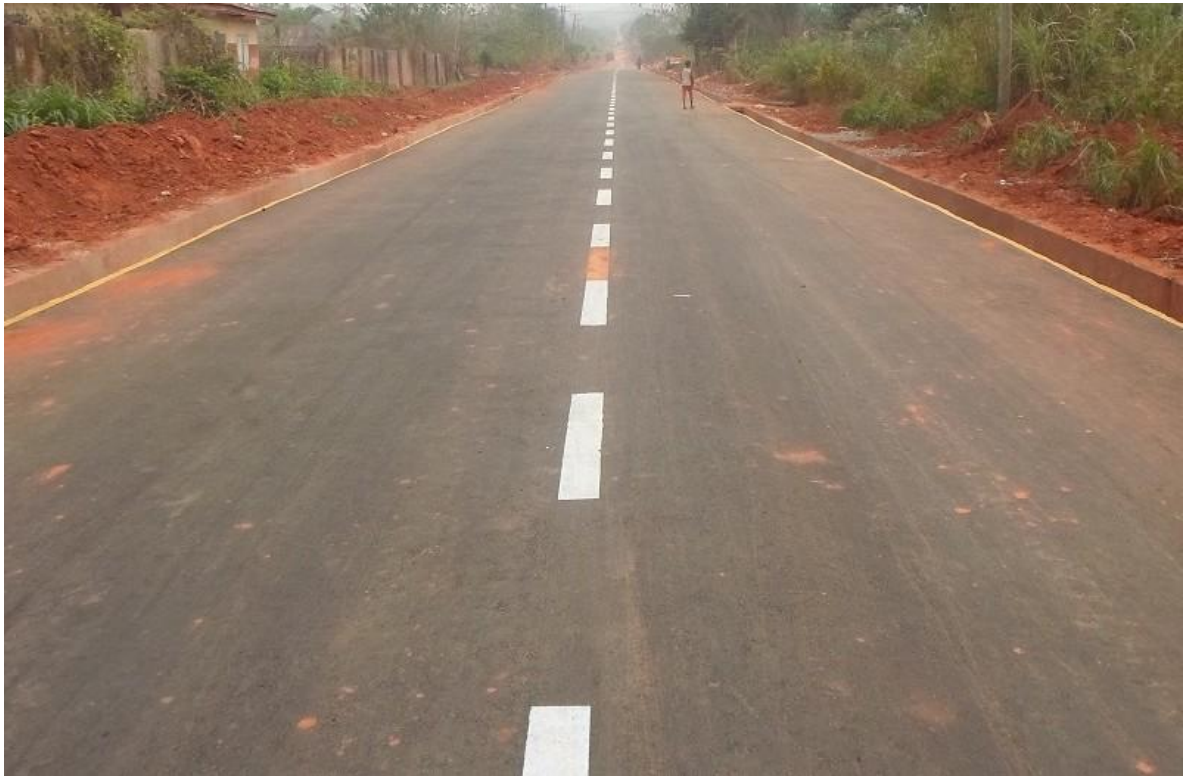
Plate 2.3 Camber, Kaduna-Kauru Road (A236)
