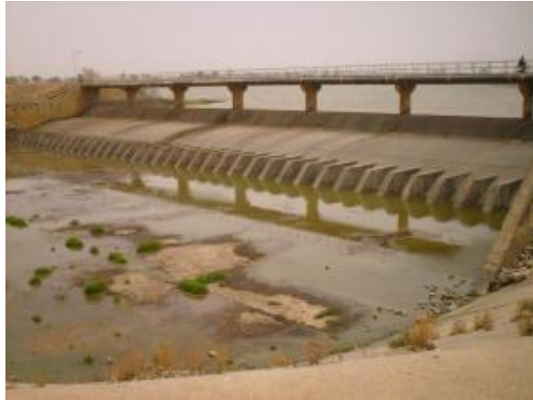
Plate 5: Kangimi Dam at Igabi local Government Area in Kaduna state. Source: Field Study, (2010).
