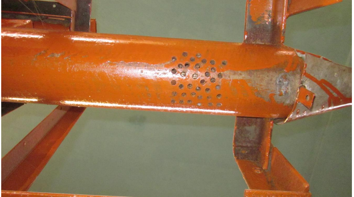
Plate C4: Photograph of perforations below the cylindrical barrel
