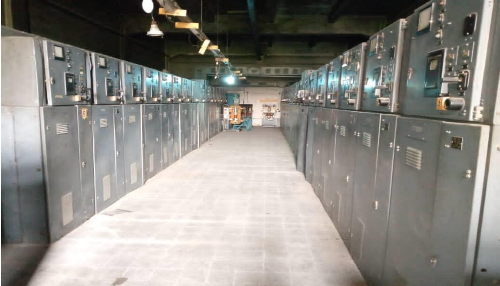
Plate 3.1 Overview of 7DS Substation
