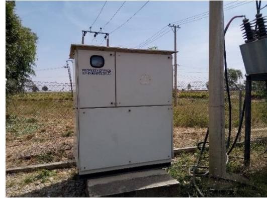
Plate II: 33KV Metering unit for ABUTH, Shika
