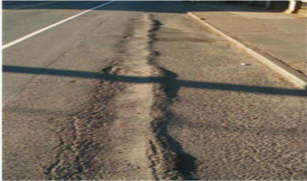
Plate IV: Permanent Deformation in Asphalt Pavement Source: Taher (2011)
