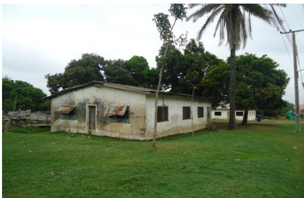
Plate 4.9 A Dilapidated Staff House in BSU
