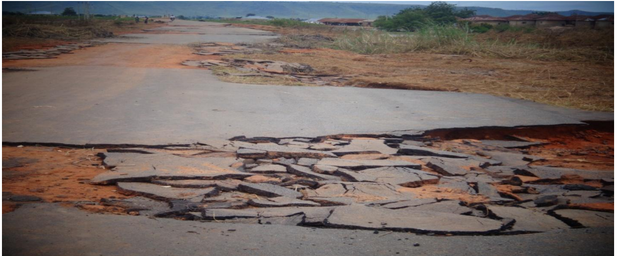
Figure 4.5: A very dilapidated portion of the road that requires complete rehabilitation
