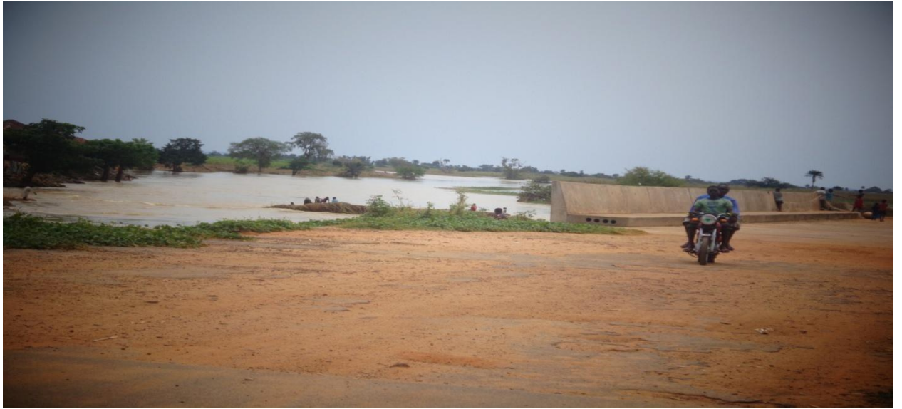
Figure 4.8: A small bridge found along the road that is almost submerged in water
