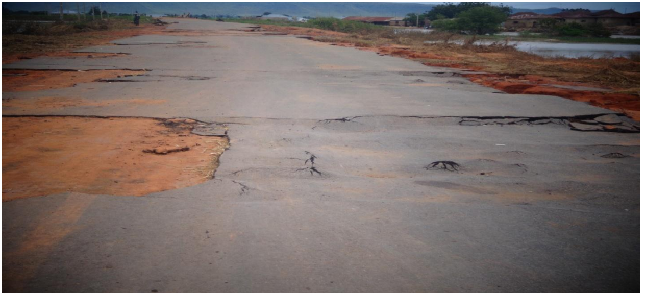
Figure 4.7: A continuing decay of the pavement of the road
