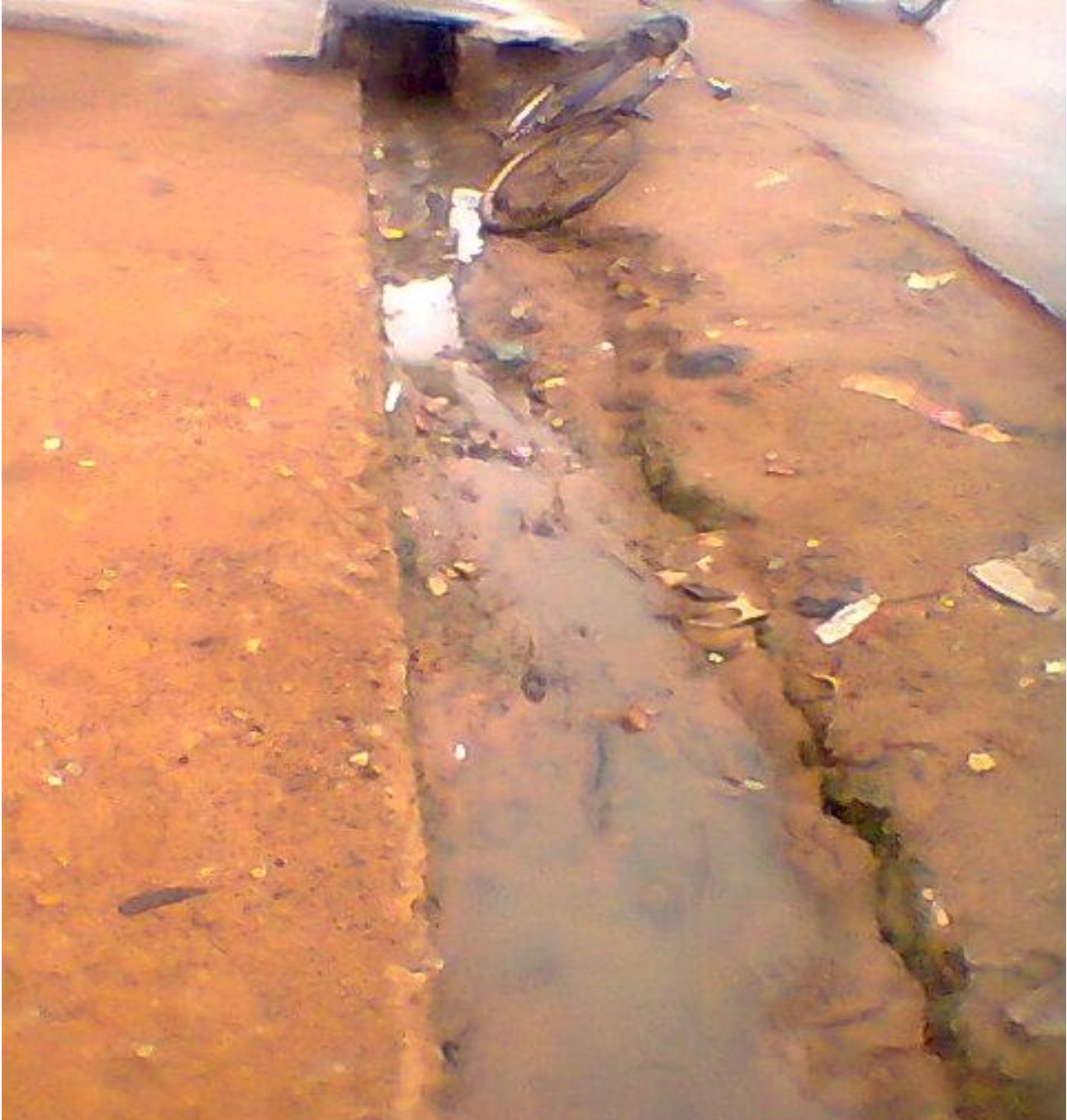
Plate 4.3: Narrow and dilapidated drainages in Henshaw town Source: Author's survey (2014)
