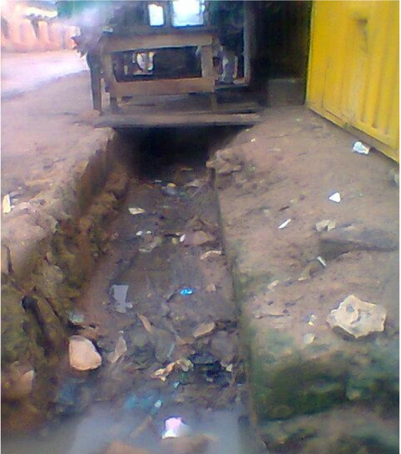
Plate 4.4: Waste dumped in drainage channels in MCC. Source: Author's survey (2014)
