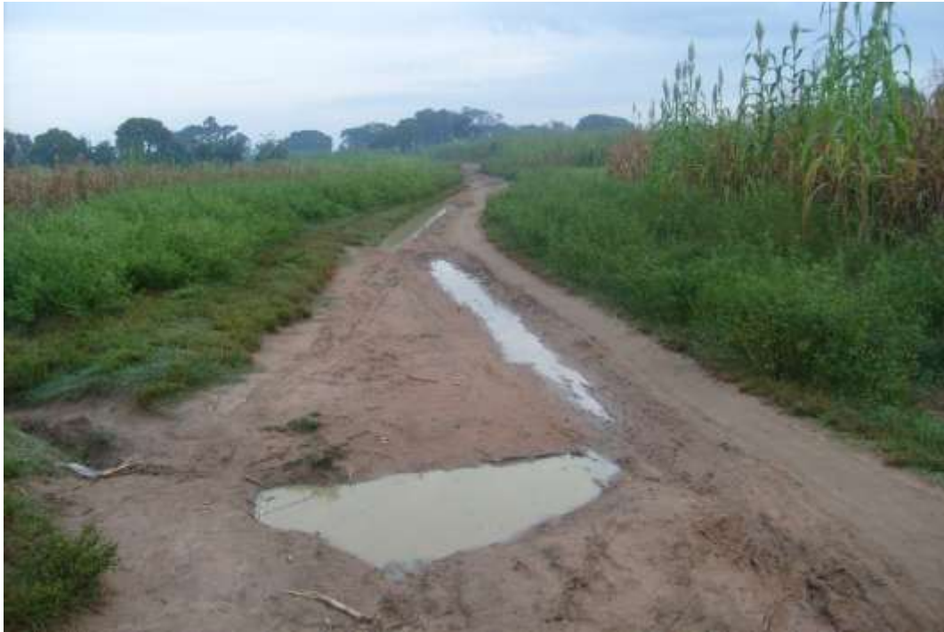
Plate III: Condition of untarred road during the rainy season along Garu to Doka Source: Authors Field survey, 2014
