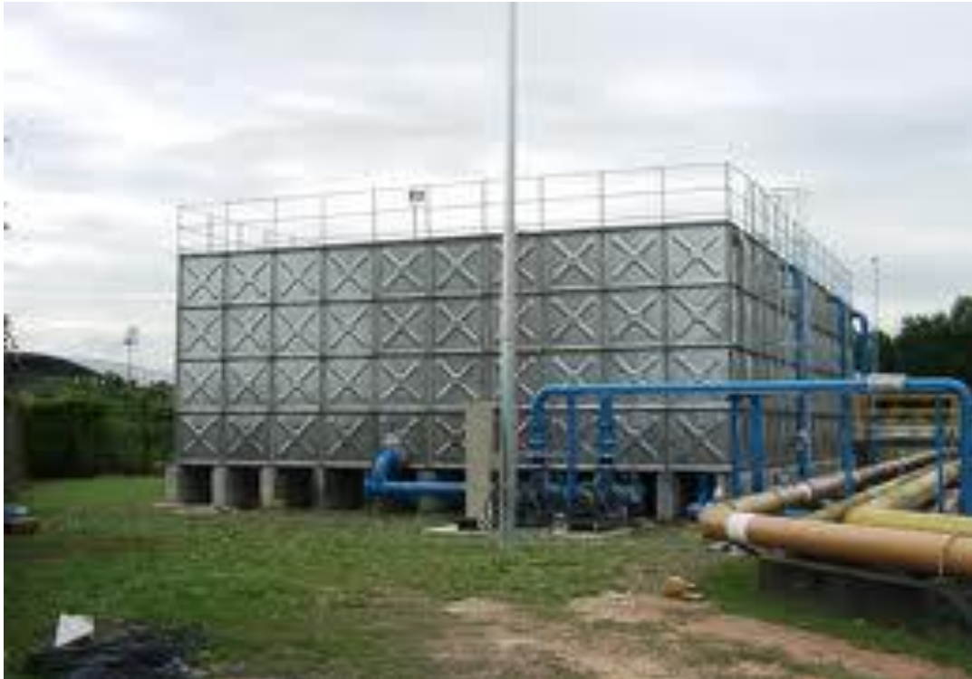
Plate 2.2: A galvanized steel water storage tank.
