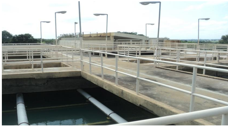
Plate 3.1a: ABU water treatment plant
