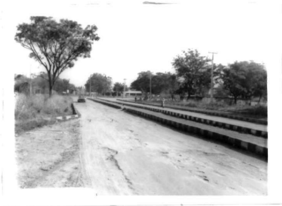
Plate 4.1. - Bad Condition of Road.
