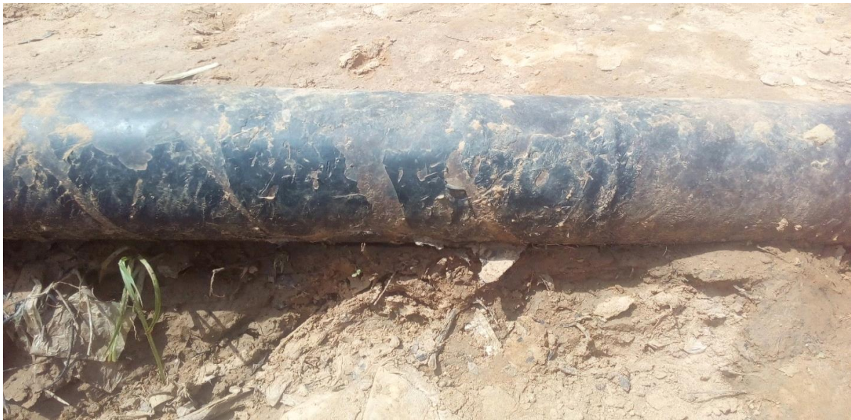
Plate 2: unbury oil pipeline interference by third- party within Hayin Mahauta community
