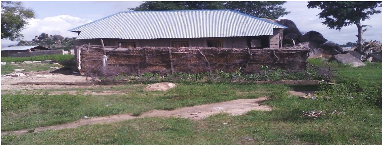
Plate i. Part of building that collapse at Tirwun. (Source field survey 2015)
