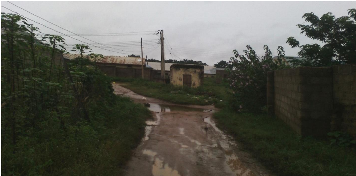
Plate xv: poor road without drainage. Source field survey 2015.
