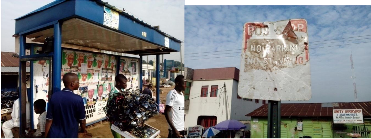
Plate: 5 shelter without passenger information Bosso route (Mobil stop) Plate: 6 worn-out pole flag (Mobil bus stop)
