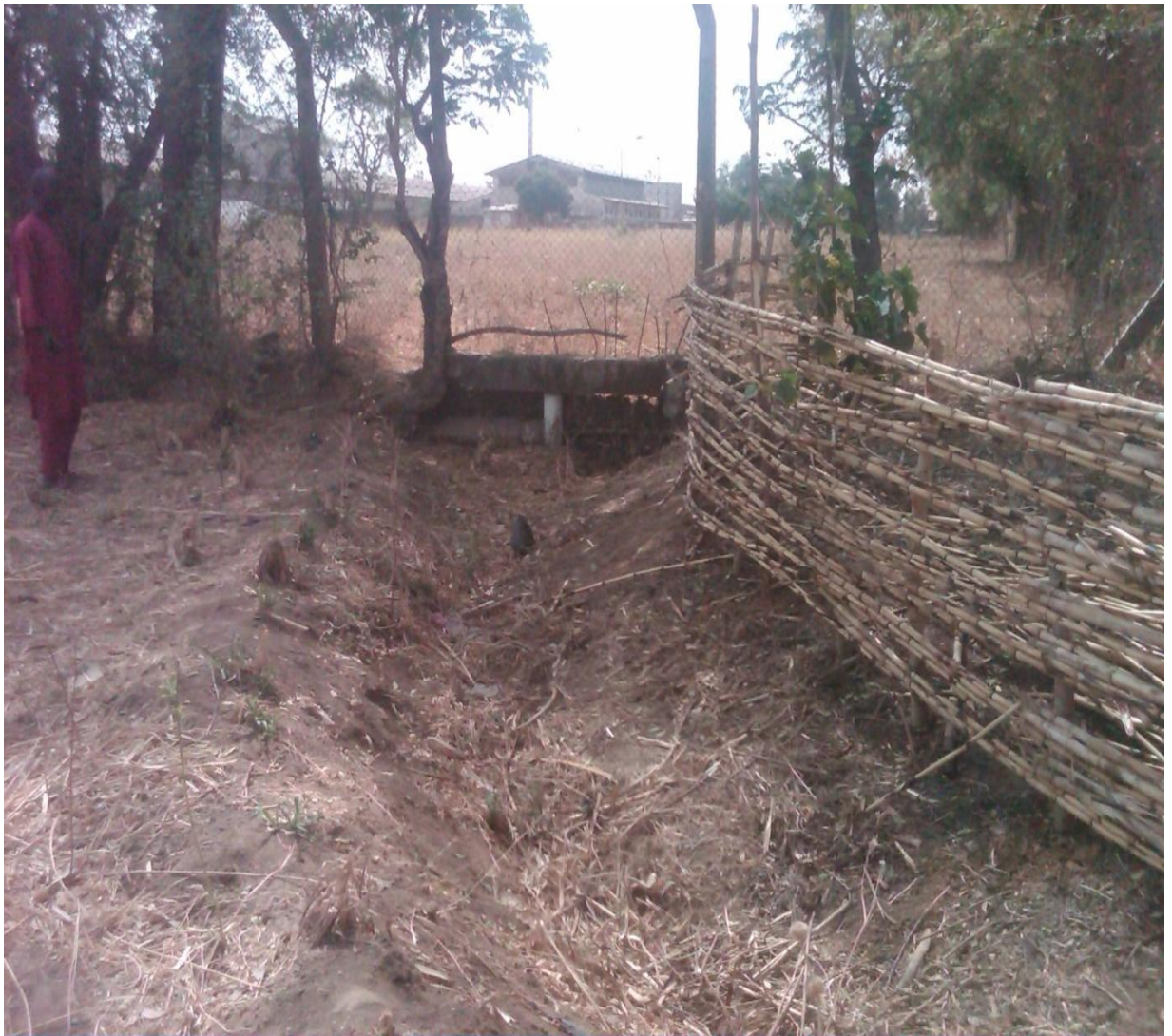
PLATE VI: Previous effluent channel from ZIL to farm lands/streams within the 20km radius of ZIL at Dakache (poor management practice).
