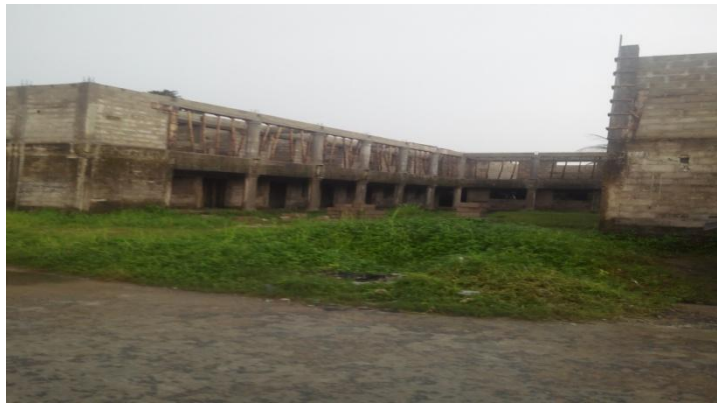
Construction of Erema Multi-Purpose Building Complex which was decided by the community to foster Youth empowerment after the TFD Intervention done in the community
