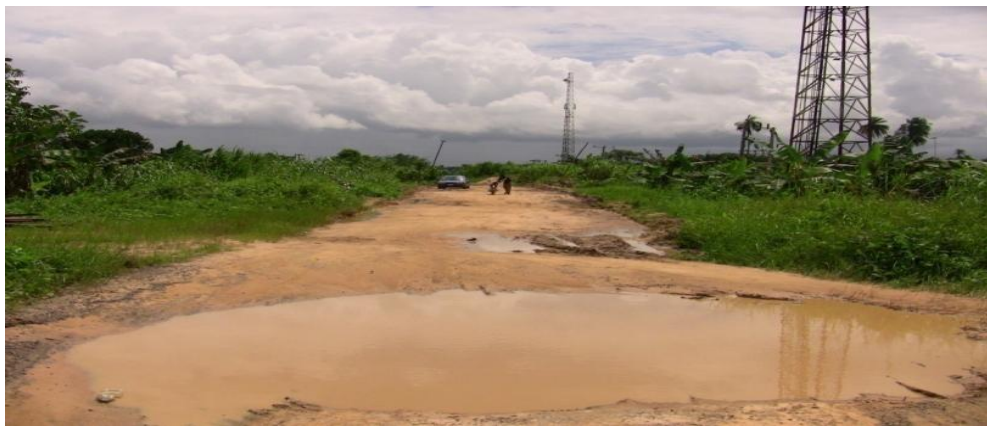
Abandoned Highway road project in Otusega Community
