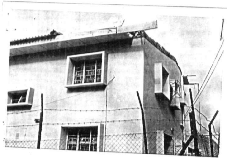
Figure 14: A four bedroom duplex with roof structure blown - off at wuse
