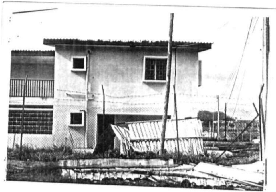
Figure 13: Aluminium sheets and purlins blown off living the rafter in position
