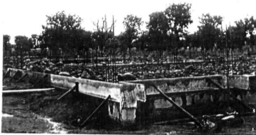
Figure 4b: Formwork ready for casting but not well braced
