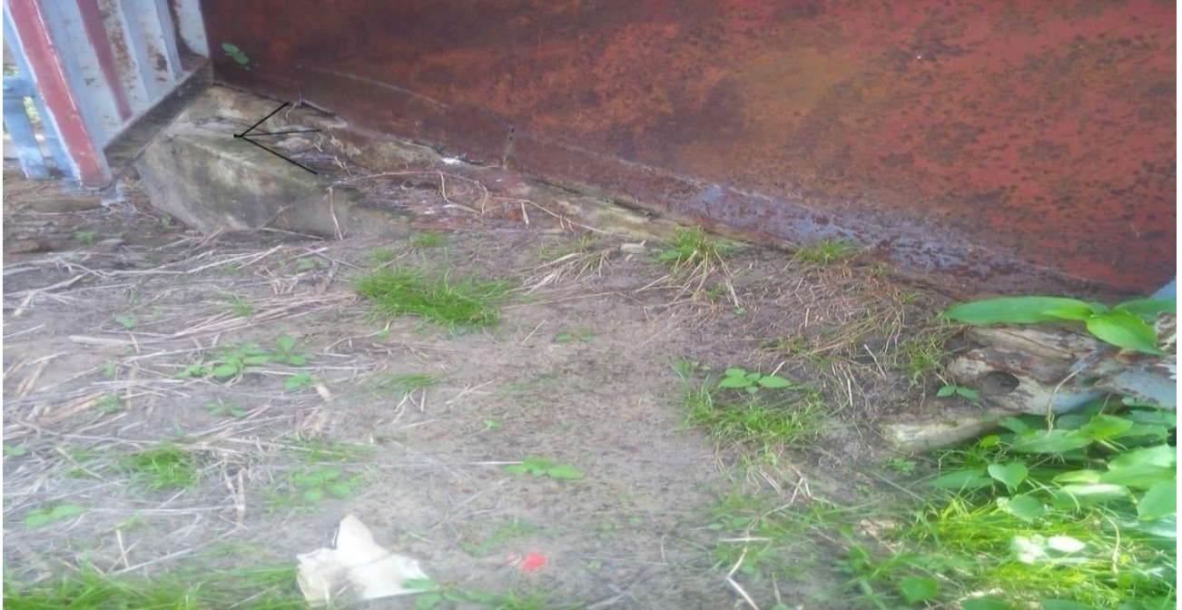
Plate V: Chemical Water Seeping of a Chemical Processing Room at Premier Seed
