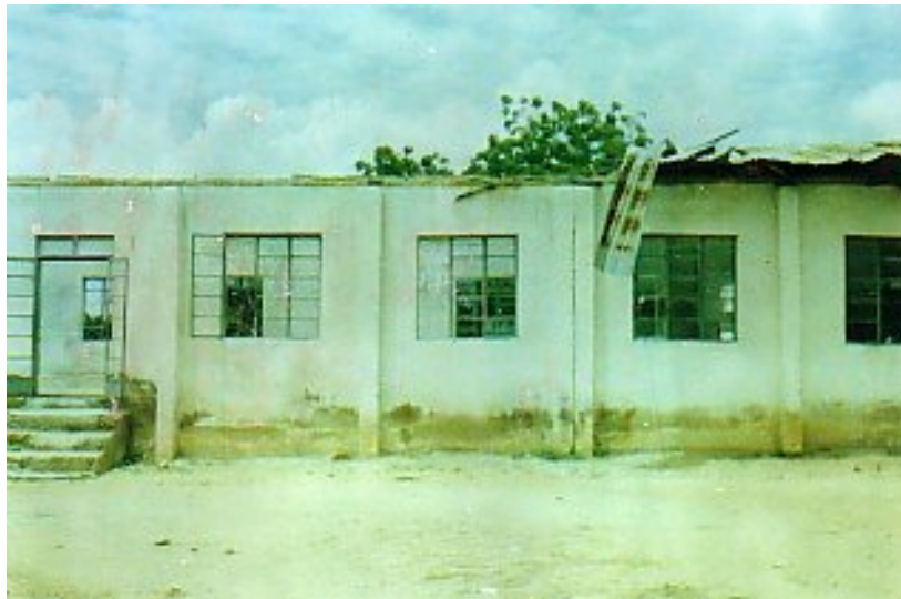
Classroom block blown by wind
