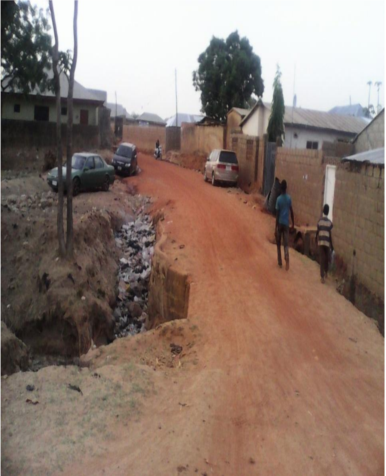
Plate XI: Gully erosion threatens the main road at Ungwan Danyaro.
